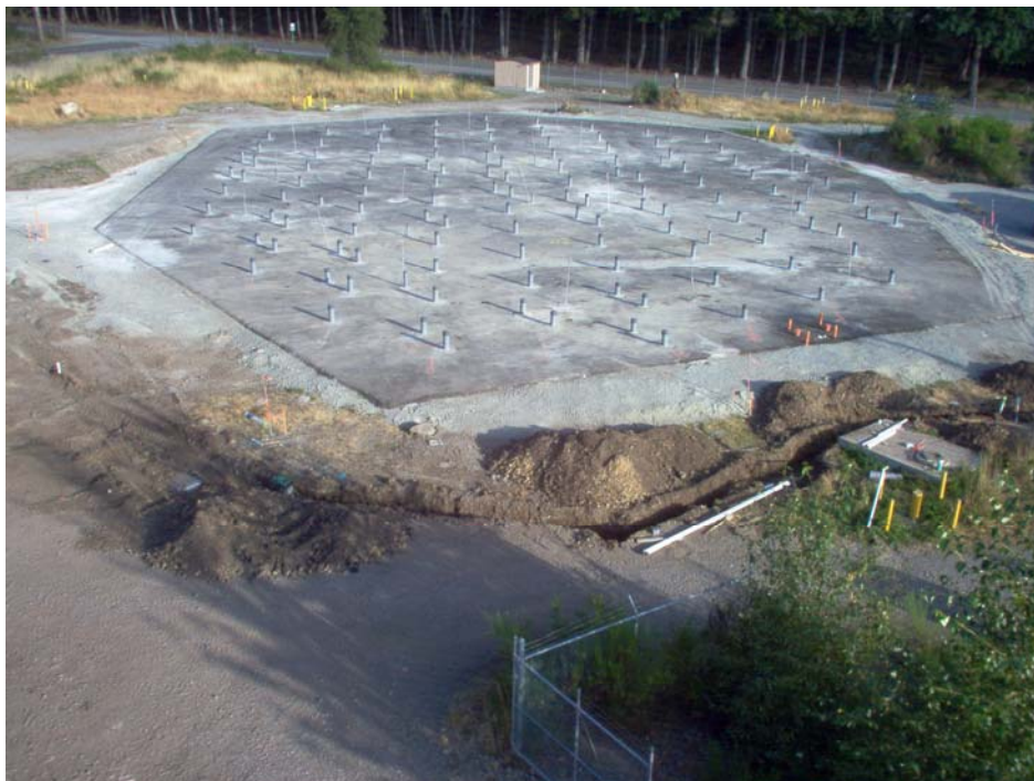
Figure 10. Electrodes Installed in NAPL Area 3
