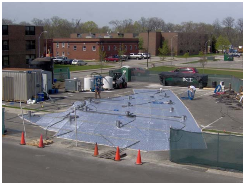
Figure 2. ERH system and related components during operation.
